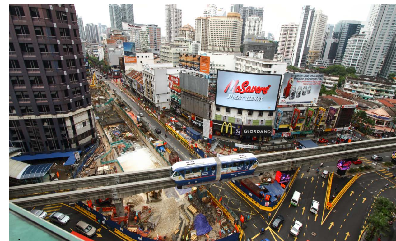
Constructing in an bustling city centre, we ensured business and utility services continuity in the area.
