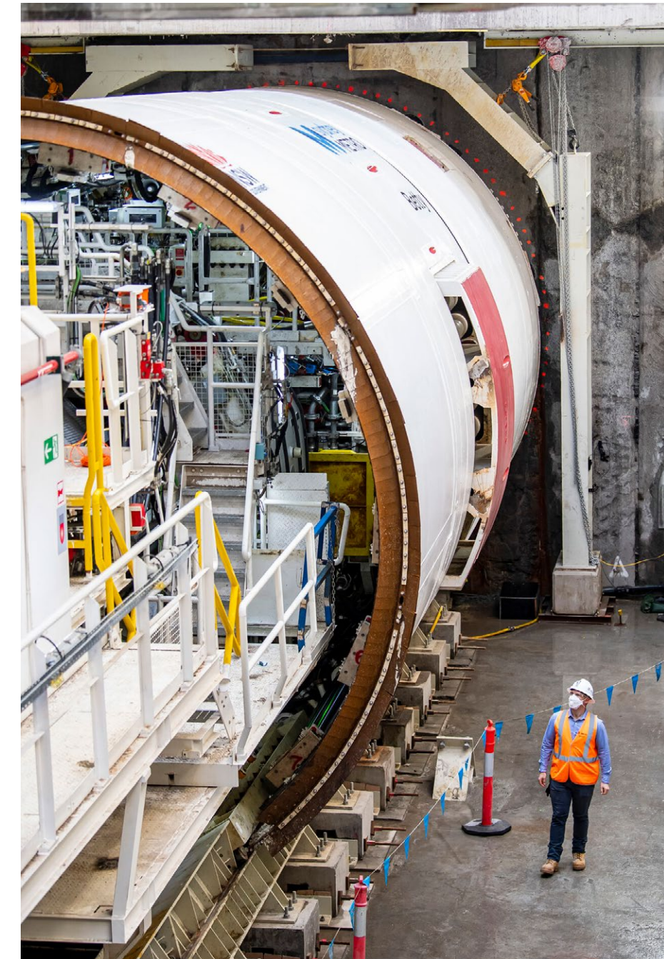
Gamuda launched TBM Betty and TBM Dorothy, Australia's first autonomous tunnel boring machines. For the first time in Sydney Metro history, TBMs Betty and Dorothy will use non-potable water to excavate and cool themselves.
